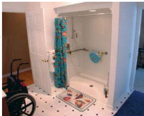
The prefabricated curbless shower has an adjustable-height bar for the hand-held shower and a lever-handled faucet.
